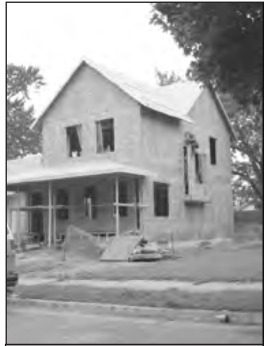
Construction continues on the new single-family house at 3028 19th Ave S. Of the three proposals solicited by the city in January -- all two storey houses -- the Housing Committee and 19th Avenue neighbors considered this one the best architectural fit for the block, which is mostly comprised of 1-1/2-storey bungalow-style homes. Local contractor D & J Steele is building the house for its future owner-occupant.
